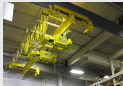
Louden crane with Speedway hoists.
